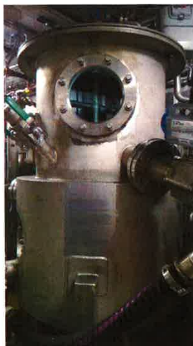
Fig. 1 The bioreactor of the ABOVE Biorefinery Pilot A
