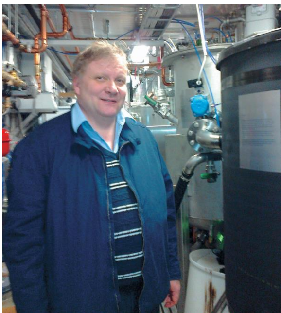
Adj. Prof. Elias Hakalehto at the final phase of the preliminary testing of ABOWE Pilot A at Savon Sella waste water treatment plant in April 2014.
