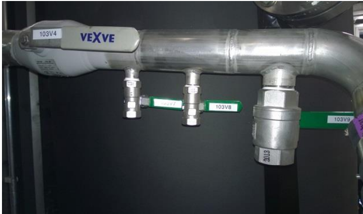
Picture 7 Circulation valves
