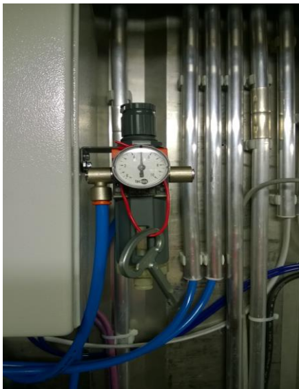
Fig. 3 Adjusting air pressure for gas mixer.
