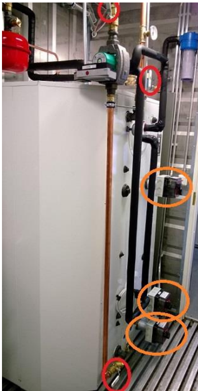
Picture 4 Water heater
