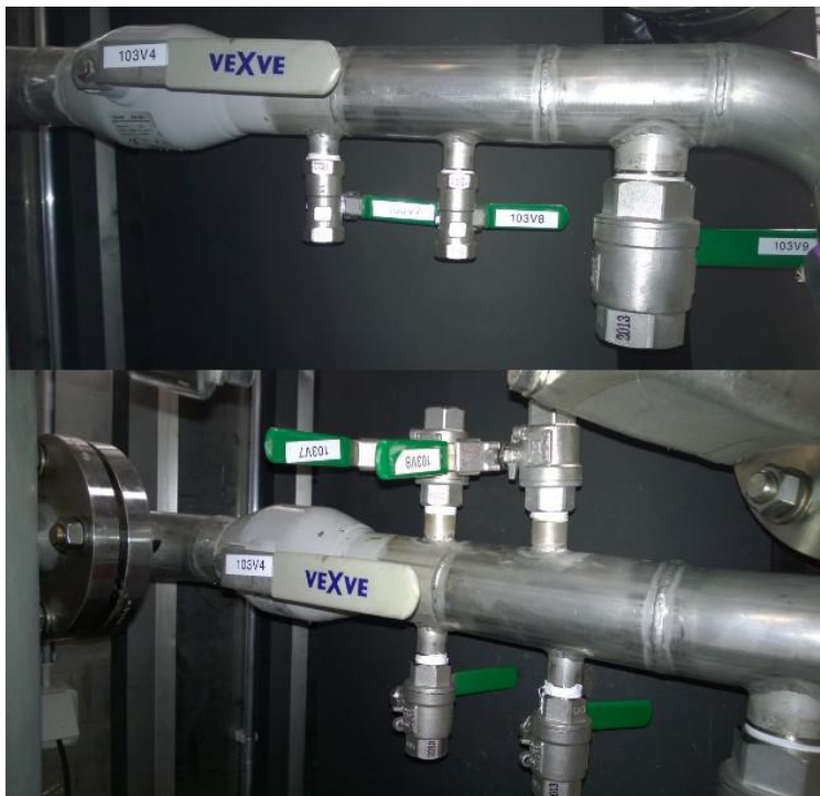
Picture 23 Upgraded pH adjusting system.
