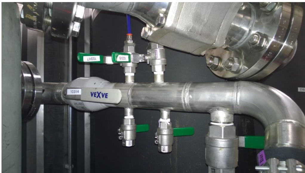
Picture 18 Reactor's circulation tube.
