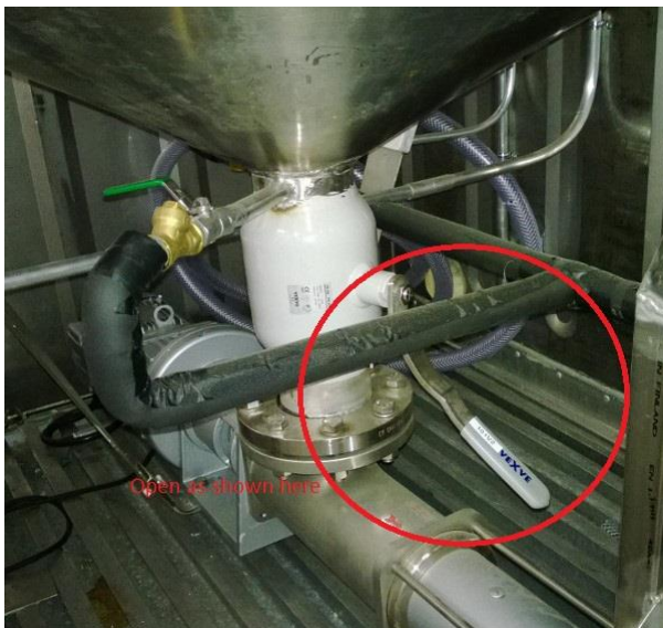
Picture 3 Valve 101V2 open
