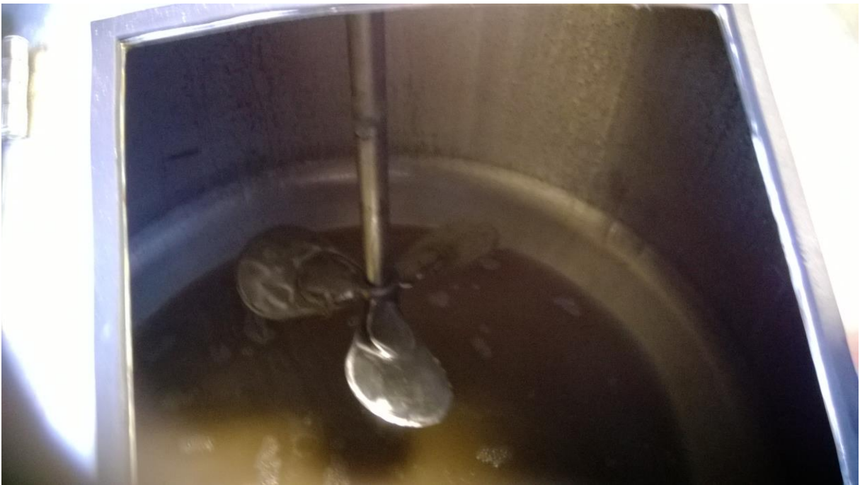
Figure 6. Waste water in the Homogenizer tank of Pilot A.
