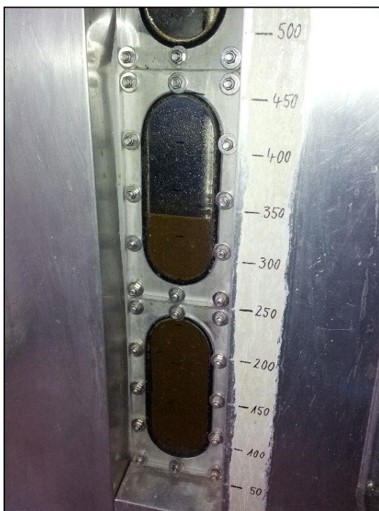
Figure 33: The fermenters level indication windows
