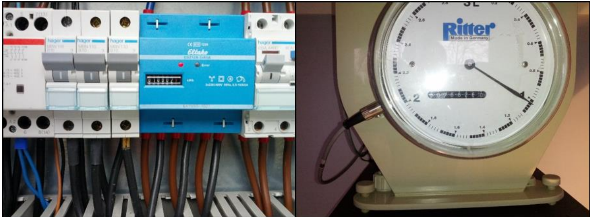
Figure 32: Electric meter in the electric cabinet outside of the fermenter (left) and gas counter inside the container (right).
