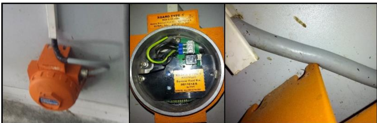
Figure 50: H 2 S-sensor from the gas warning system. Sensor had a closed circuit, causing false alarms.
