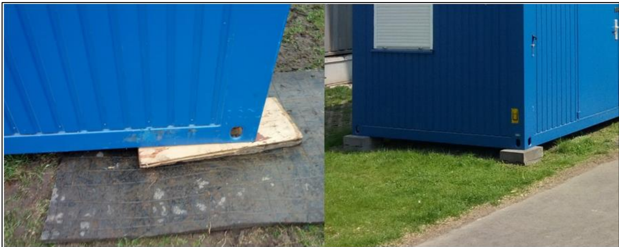
Figure 25: Leveling of the container with wooden boards (left). The rubber mat provides a large supporting surface. Leveling with flagstones (right).
