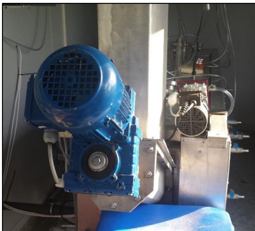
Figure 12: Motor of the screw conveyor.
