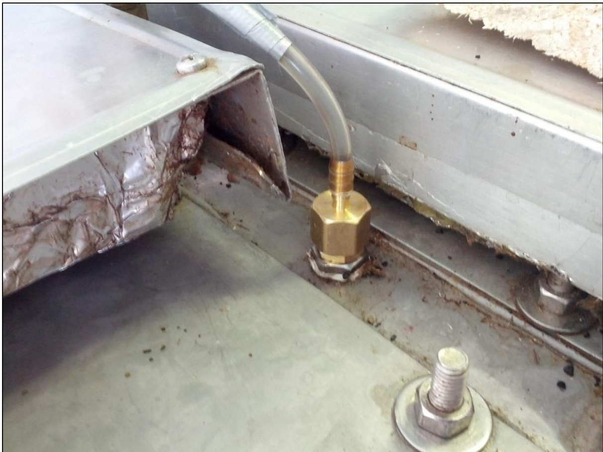
Figure 53: Gas outlet for the gasmeasuring system. Due to clogged openings by condensate they have been exchanged to outlets with a bigger diameter as shown in the picture.
