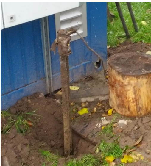
Figure 27: Metal stick for grounding of the container.
