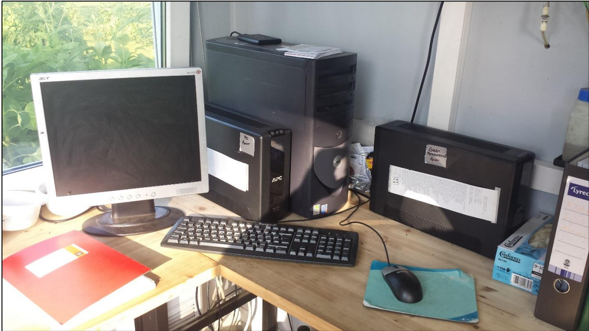
Figure 18: Desktop computer for plant control. The two black boxes (right and center) provide emergency power supply for the computer and the gas measurement system in case of a blackout.
