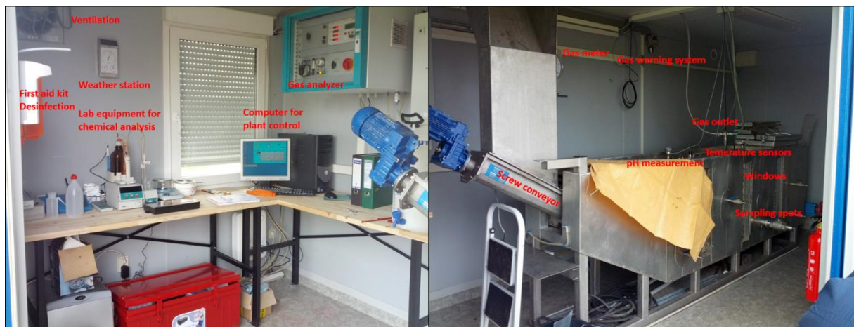
Figure 2: Interior of Pilot B Container. Left side: Laboratory, plant steering and measuring equipment. Right side: fermenter with technical equipment.
