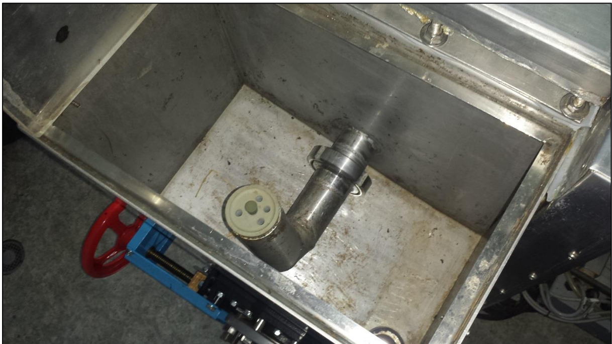
Figure 3: Overflow box at the end of the fermenter. In the center the pipe bend DN 50 to adjust the overflow level.
