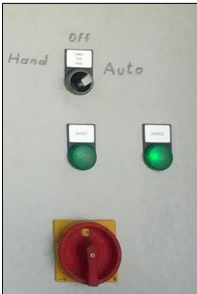
Figure 23: Switch on the main electric cabinet to choose between manual- and auto- mode. Below the plants main switch.
