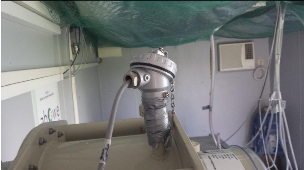
Figure 54: Sealed leakage at the thermometer of the gas clock. Sealed with glue and sticky tape.
