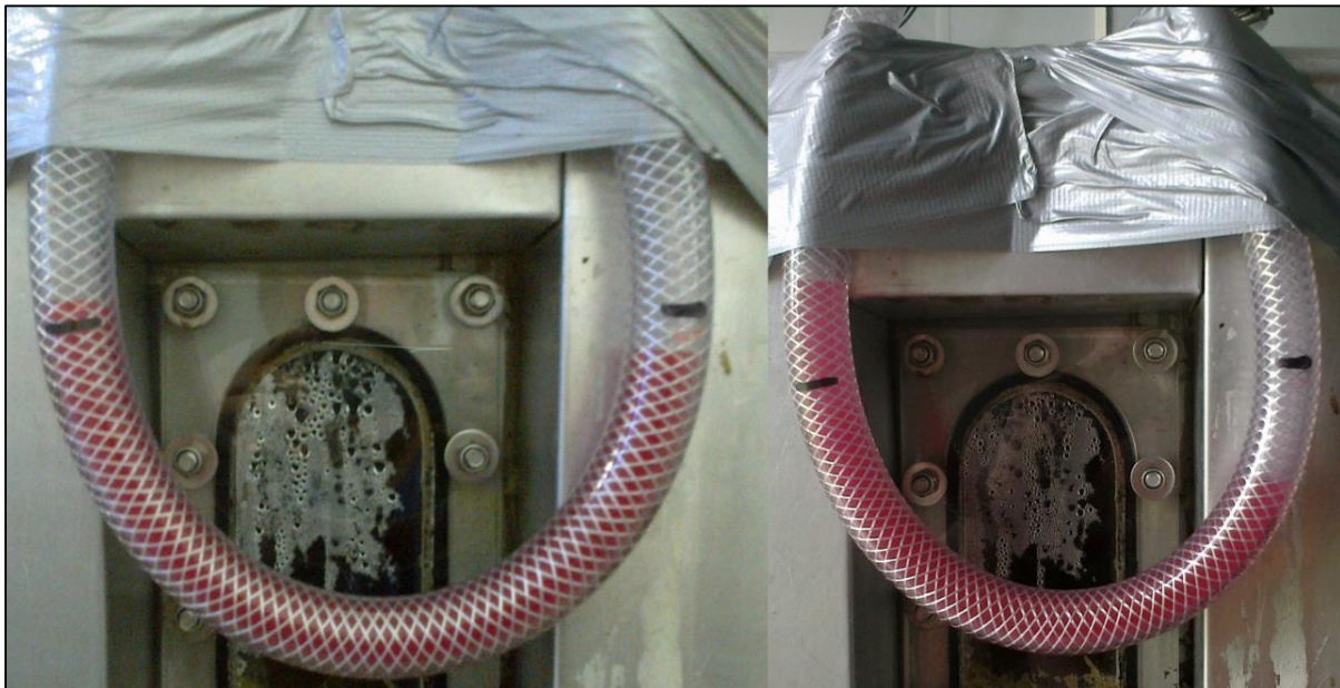
Figure 49: Improvised u-tube manometer connected to the main valve. Pressure balanced (left). Overpressure (right).
