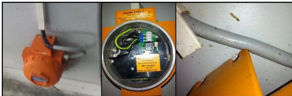
Figure 25: Broken H 2 S-alarm-sensor, caused by closed circuit in the sensor.
