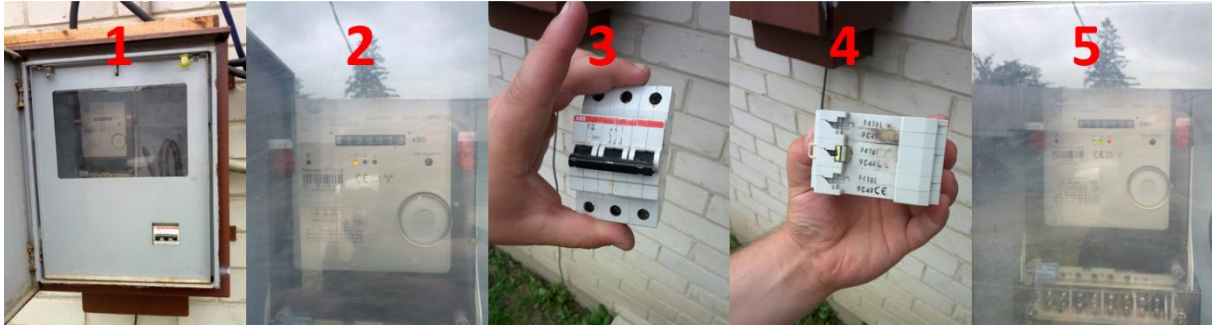
Figure 26: Damage caused by lightning strike to the electrical grid. (1) farms` main electric cabinet, (2) electric meter with only phase L1 showing light, (3) + (4) broken main fuse, (5) electric meter showing light on all phases after repair.
