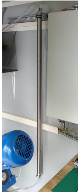
Figure 24: Activated carbon filter for H 2 S-elimination from the biogas.
