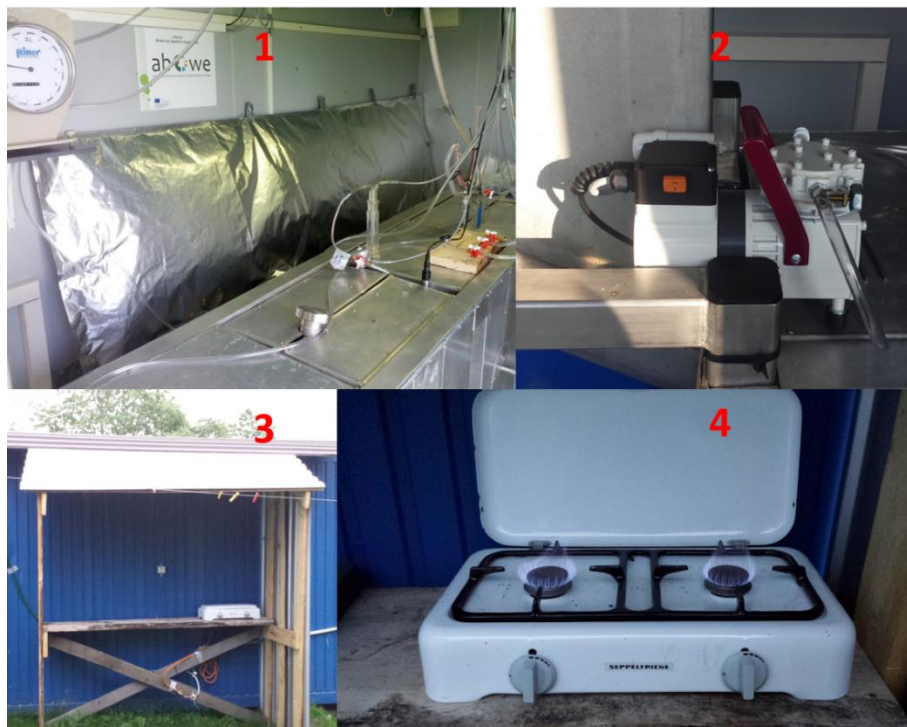
Figure 21: Pilot B gas utilization: (1) one of three 250 liter gas bags, (2) gas pump, (3) outdoor kitchen, (4) 2-flame gas cooker
