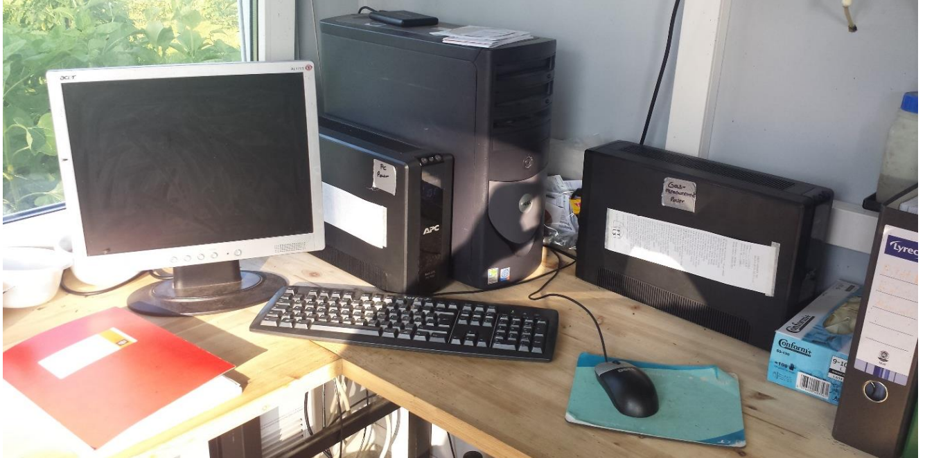
Figure 6: Emergency power supply kits for control-computer and gas measurement system
