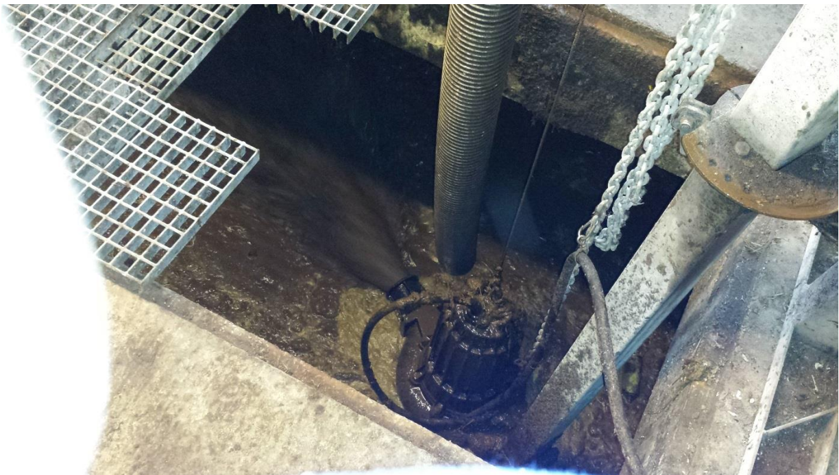
Figure 3: Slurry pit at Karlii Farm OÜ
