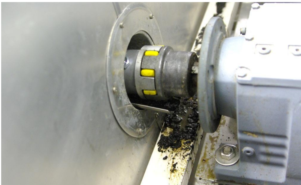
Figure 11: Leaking stirrer No. 3.
