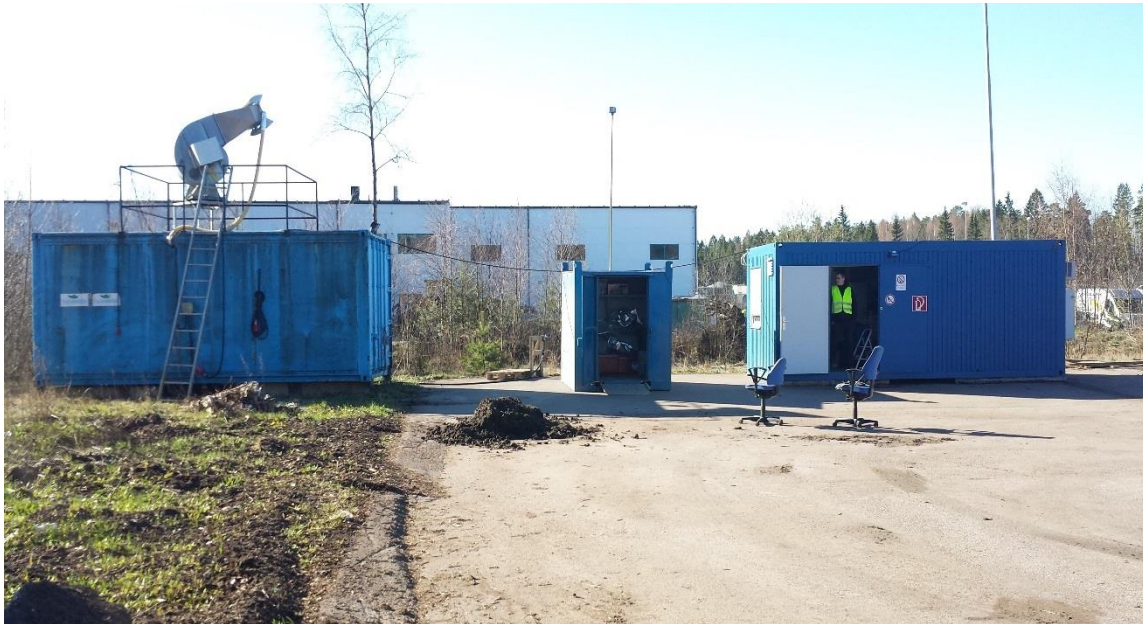
Figure 5: Connecting the pilot plant to the local electric grid.
